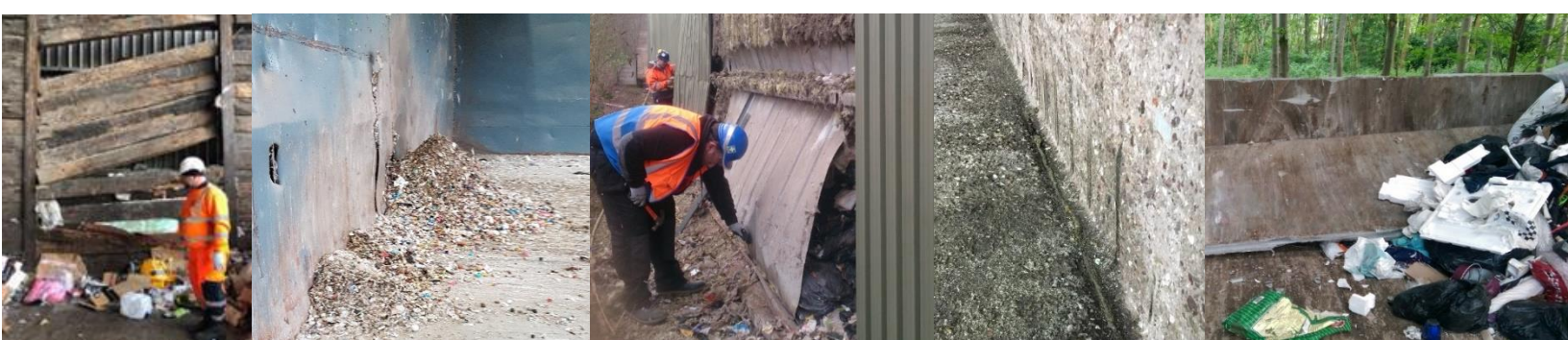
Examples of damaged and collapsed walls
