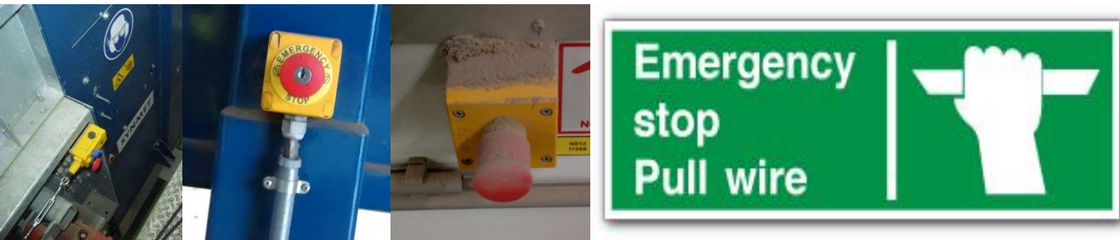
Left to right: Switch at one end of a pull-wire stop on a conveyor, keyed button emergency stop, dusty stop – likely not been tested recently (plus dust ingress can cause stops to fail, typical signage for a pull-wire emergency stop)
