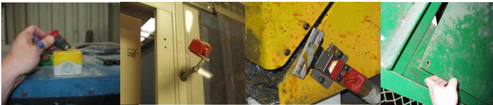
Left to right: damaged emergency stop, non-robust fixings (self-tapping screws) resulting in an interlock pulling free of its mounting, deliberately tampered with interlock, damaged fixed guard (bolt fixing sheared)
