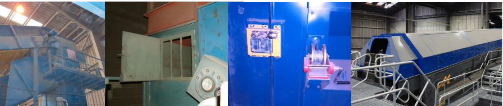
Left to right: Access platform at the top of a baler feed chute, jailers bars fitted at an access hatch, winch mechanism operating a drawbridge to allow safe access to a screen, trommel screen with gantry and door access
