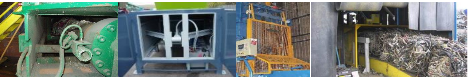
Left to right: inadequately guarded rear of baler ram (crawl access at the side possible), example view rear ram area (hinged guards open), baler wire needle area with large mesh guard fitted, bale ejection area with interlocked sliding guard over needles and bale wire-tie mechanism
