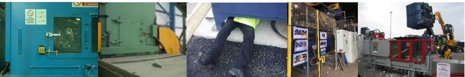
Left to right: two examples of interlocked access doors to baling chambers, inadequate guarding on a baler – well guarded from above but access possible underneath, example of perimeter/machine fencing at a baler, example of a smaller direct feed baler
