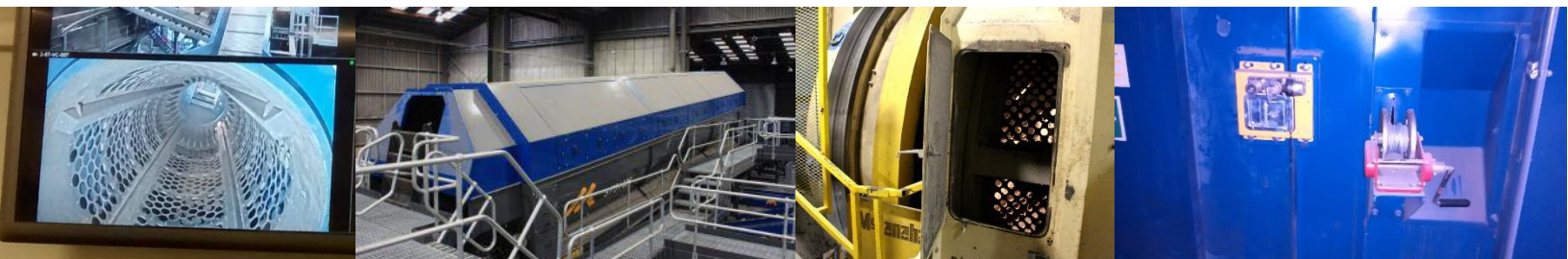
Left to right: CCTV installed in one end of a trommel screen to provide operatives with a view of what a problem might be before entry is attempted, large enclosed trommel with access door at one end, access hatch into a trommel screen, winch mechanism for a 'drawbridge' system allowing safer access across the output chute of a trommel
