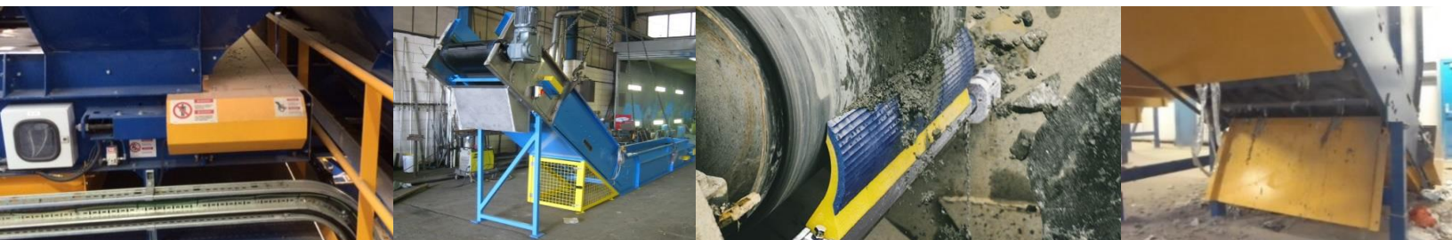
Left to right: fixed guard designed to allow belt tracking without removal, example of a drop-out chute (in this case with an interlocked gate access to clear debris), example scraper bar (guard removed to show detail), example hinged guard at a conveyor tail roller to make cleaning easier for operatives
