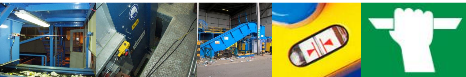
Left to right: pull-wire emergency stop above a conveyor (in this case with a non-compliant fixed mounting at one end), typical switch at one end of a pull-wire, load conveyor to a baler fitted with goal post pull-wire emergency stop system above the conveyor, typical tension adjustment window – line between the arrows, pictogram signage for a pull-wire
