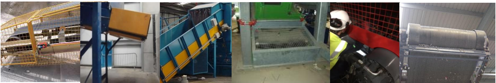
Left to right: mesh fixed guard at tail roller, fixed close guard at tail roller, drop-out chute to reduce detritus build-up, large mesh guard at tail roller, inadequate guarding allowing reaching access, nip/finger guards at head roller
