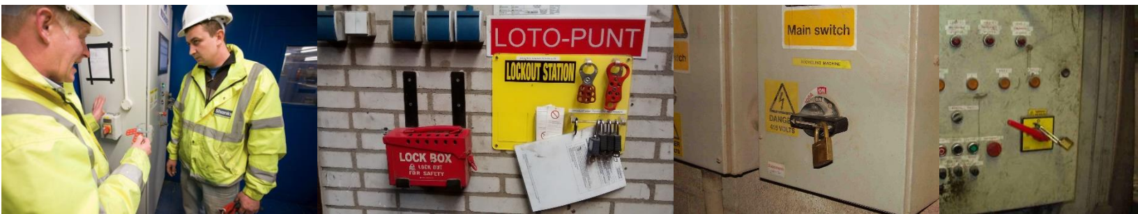
Left to right: Isolation/lock-off training at a recycling plant, example lock-off station (note – 'LOTO' is another term sometimes used for isolation/lock-off – 'lock-out-tag-out'), two examples of isolation switches with lock-off padlocks inserted
