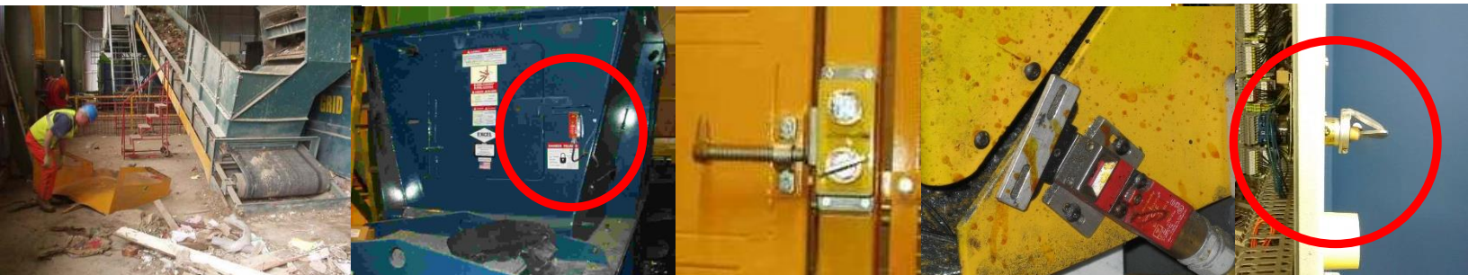
Left to right: Removal of a fixed guard at the end roller of a conveyor, interlocked access hatch in a baler feed chute, retained key interlock at a machine fence gate, defeated 'tag' switch interlock (scene of an accident – red dots are blood), retained key master key in control panel with door of panel open to show control circuit wiring behind it (that is power is not turned-off direct)
